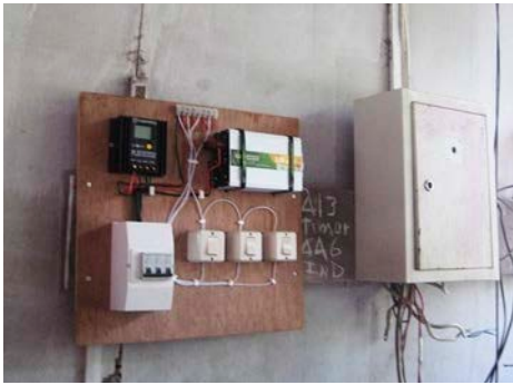
↑ The switchboard for the new system (left) sitting next to the old switchboard.
