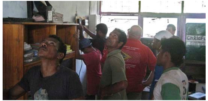
↑ Helpers running cables from the classrooms to the staff room where the switchboard was being installed.
